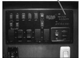
Monitor panel and command center panel
