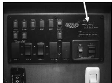
Monitor panel and command center panel
