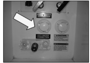
City Water/Fresh Water inlet
