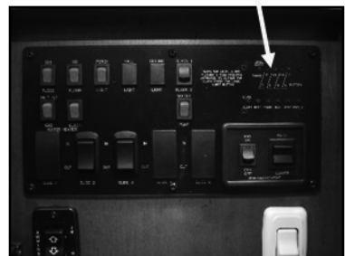
Monitor panel and command center panel
