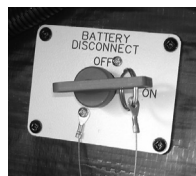
Battery Disconnect Switches
