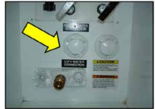
City Water/Fresh Water inlet
