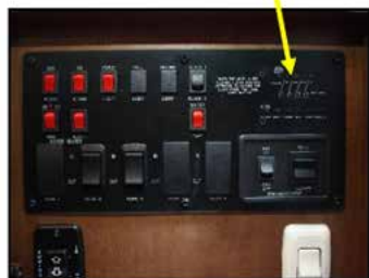
Monitor panel and command center panel
