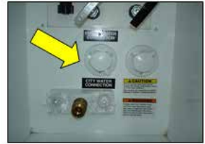
City Water/Fresh Water inlet
