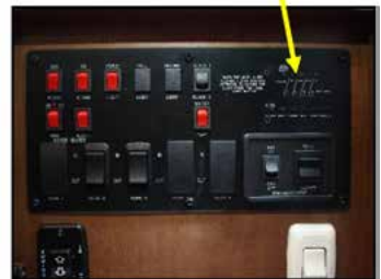
Monitor panel and command center panel
