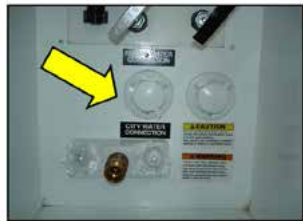
City Water/Fresh Water inlet
