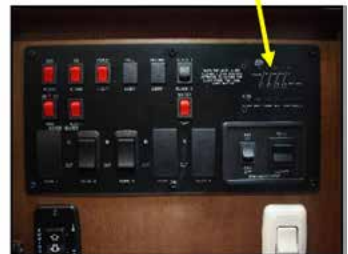
Monitor panel and command center panel
