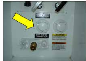
City Water/Fresh Water inlet
