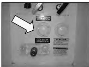
City Water / Fresh Water inlet
