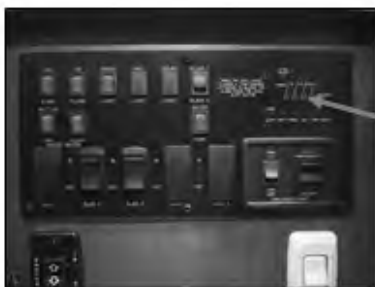
Command center panel
