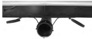
Black/Grey tank drain & valves
