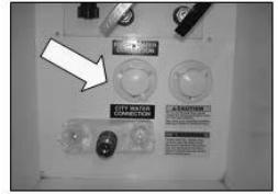
City Water/Fresh Water inlet
