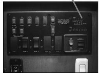
Monitor panel and command center panel
